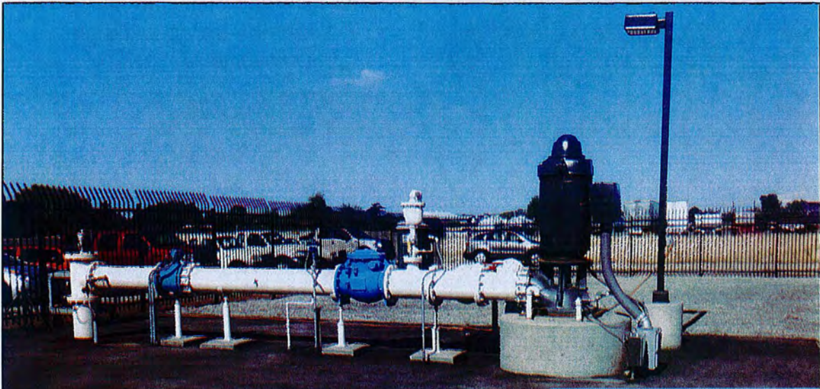
Wellhead & Connection Pipe
